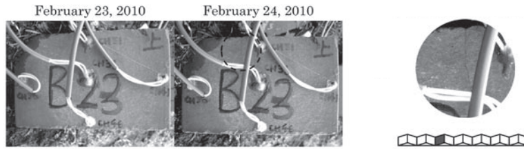
Fig.24 Crack of the brick No.3 that occurred at (a) Snow removal (Picture taken on February 23 & 24, 2010) .
