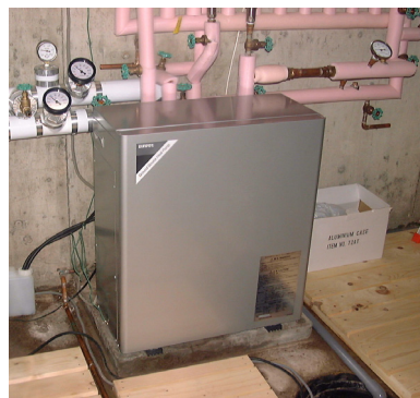
Fig. 2 GHP unit installed at the basement
