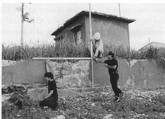
Photo. 26 Crack and deteriorated part of coastal revetment of the structure
