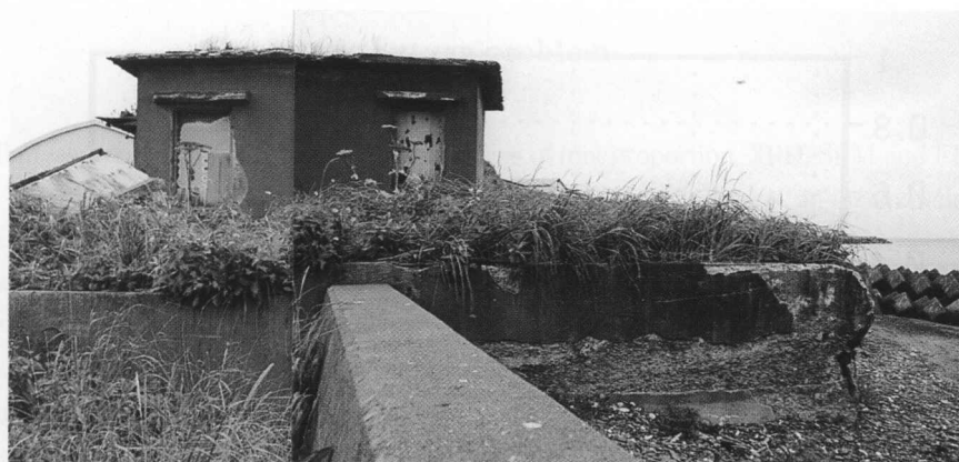
Photo. 24 Coastal revetment surrounding the structure, which is estimated to have been constructed at the same time, but this side is the present days.
