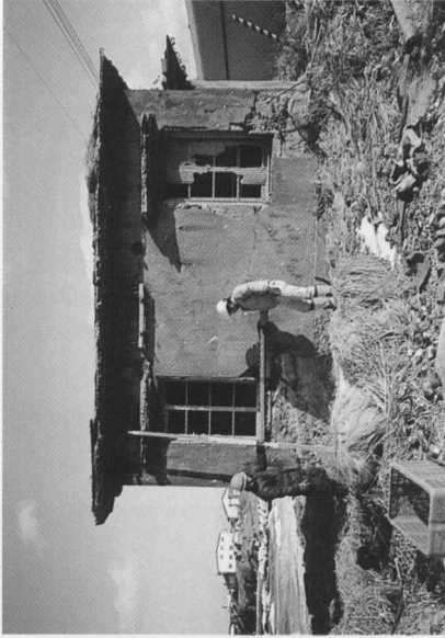
Photo. 11 The west side which is deteriorated due to many cycles of freeze and thaw with sunshine in the afternoon in winter
