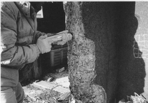
Photo. 18 Low repulsion of deteriorated part
