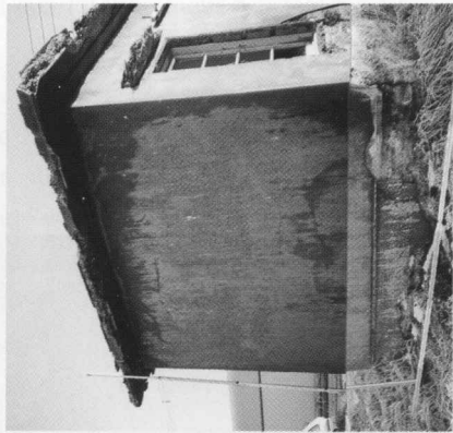
Photo. 12 The north side which has deteriorated comparatively light
