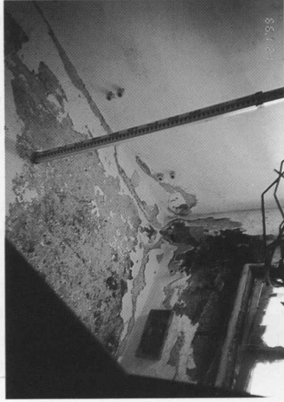
Photo. 23 Plaster finished wall and plastered ceiling at the west side in cable-pit room where insulators are installed.
