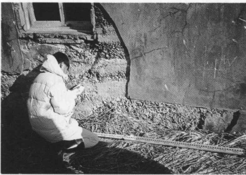
Photo. 27 Delaminated mortar finish and building frame concrete on exterior wall face at the west side
