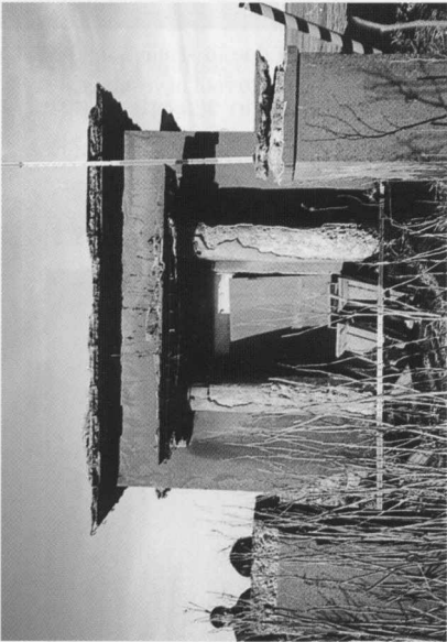
Photo. 10 The south side which has deteriorated due to many cycles of freeze and thaw with sunshine in winter
