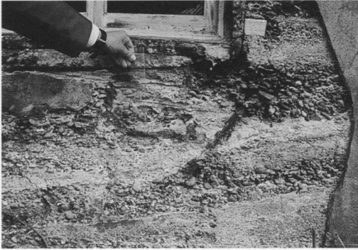
Photo. 16 Corrosion of steel in shallow depth under a window on the west side
