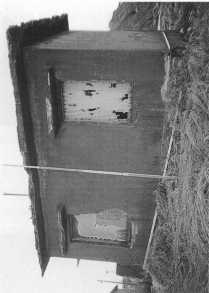
Photo. 13 The east side which has deteriorated comparatively light
