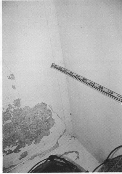
Photo. 22 Comparatively beautiful plaster and concrete on ceiling and partition wall in cable-pit room without leakage for long year.
