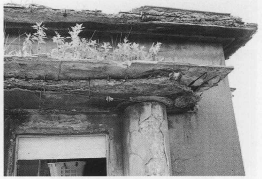
Photo. 15 Deterioration of lean-to roof of vestibule of on the south side
