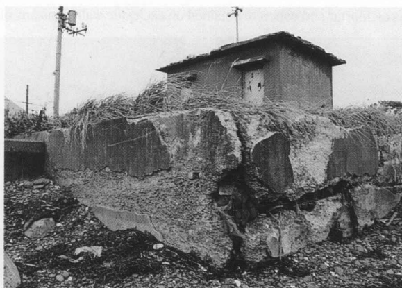
Photo. 25 Coastal revetment is reinforced concrete and stone were used as back-fill material.
