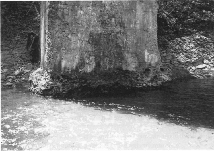
Photo. 8 Scour of the foundation at Obihiro side (1P from Obihiro side) of Dai Go Otofuke Bridge
