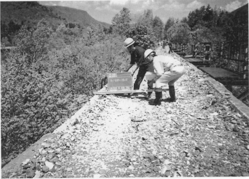
Photo. 6 A complete view of deck of Dai Go Otofuke Bridge from Obihiro side and the edge of deck is deteriorated.
