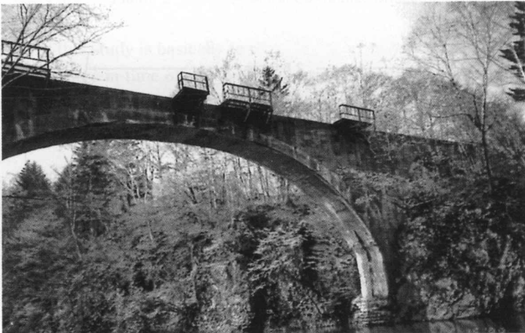
Photo. 3 The shape of Dai San Otofuke Bridge from river side and a little scour of the pier foundation at Tokachi Mitsumata side (under 3P from Obihiro side)
