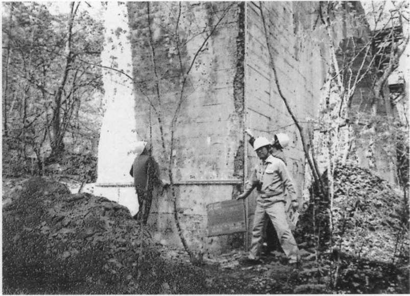
Photo. 4 Deterioration and scaling at the edge of member caused by frost damage on 2P from Obihiro side of Dai San Otofuke Bridge
