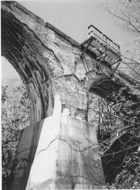
Photo. 7 Deterioration and crack at a part of repair on 1P from Tokachi Mitsumata of Dai Go Otofuke Bridge
