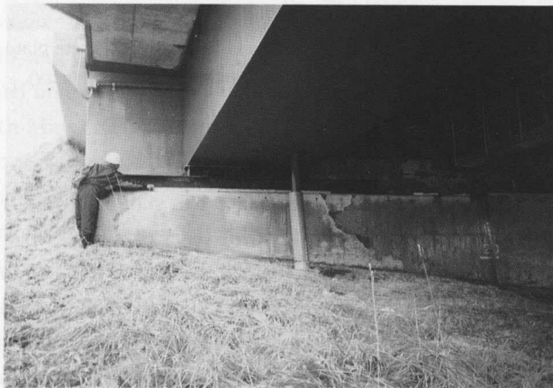
Photo 3 Failure of the anchor support, cracking, and scaling of the concrete abutment. The width of the abutment: 275 cm at the upper part and 460 cm at the lower part. (Road bridge, 3 spans continuous, 2 main girders box section, Midorimachi in Nakashibetsu town)
