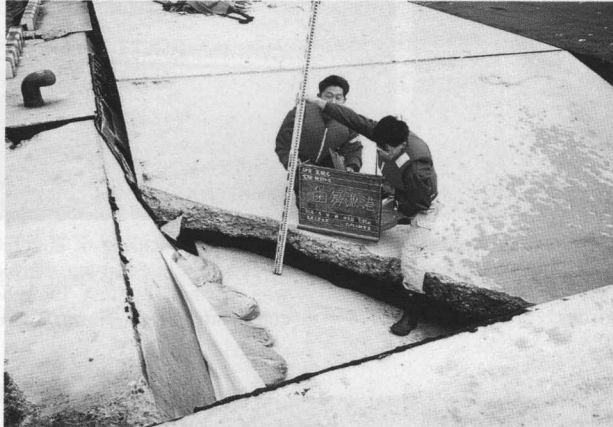
Photo 5 Wharf tilted and sunk and broke the concrete plate of apron (Fishing port, habomai in Nemuro city)
