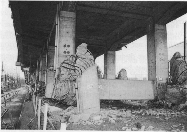
Photo 10 Concrete destroyed, stirrups failed and the longitudinal reinforcing steel yielded and deformed at recessed part of RC pier (Express railway bridge, PC girder, near Mukogawa river in Nishinomiya city)
