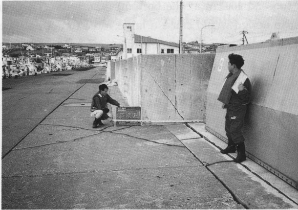
Photo 4 Cracking at the concrete base for the gates and shear cracks on the anti-tidal wave quaywall itself (Fishing port, Hanasaki in Nemuro city)
