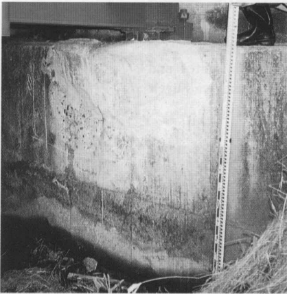
Photo 1 Failure of the anchor support, cracking, and scaling of the concrete abutment (Road bridge, composite girder, Manmen in Bekkai town)
