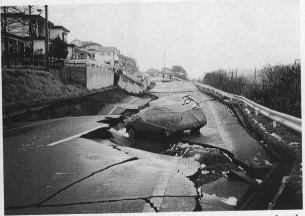
Photo 8 Collapse of a road embankment subbase caused an L-shaped concrete retaining wall to slide 3.5 m and subside by 2.5 m (at Matsugaoka in Hachinohe city)
