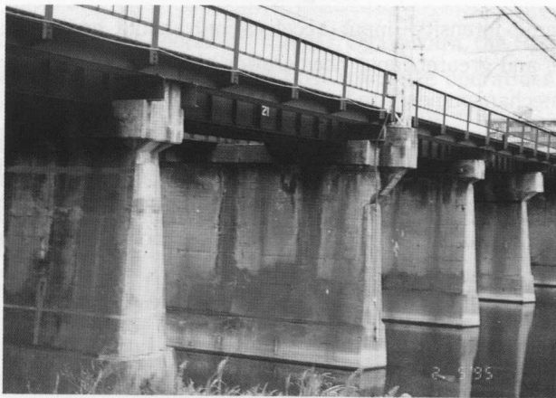
Photo 11 Undestroyed RC pier (Rail way bridge, steel girder, constructed in 1926, Mukogawa river in Nishinomiya city)
