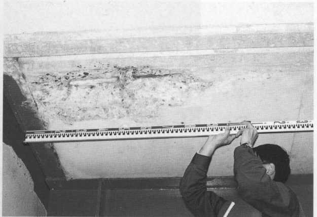
Photo 2 Failure and scaling of concrete, exposure of stirrup steel, and other damage were caused when the girder was crushed against the abutment (Road bridge, composite girder, Furen in Bekkai town)
