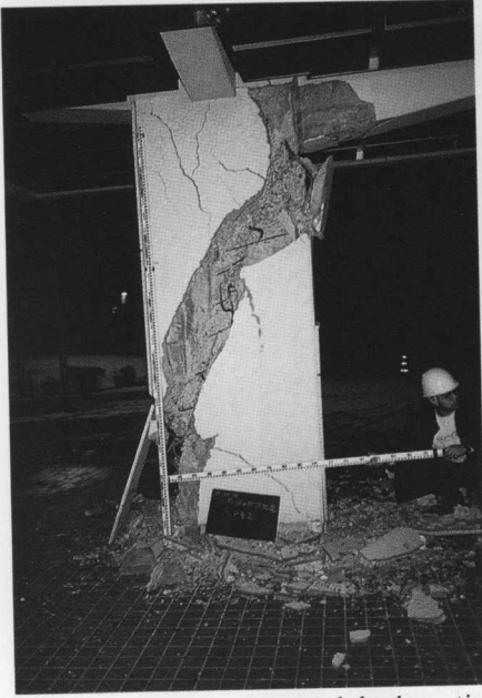
Photo 7 Concrete destroyed, broken stirrups, deformation and yield of longitudinal steel at recessed steel section past of RC pier (the first floor of 3 stories high school building in Hachinohe city)
