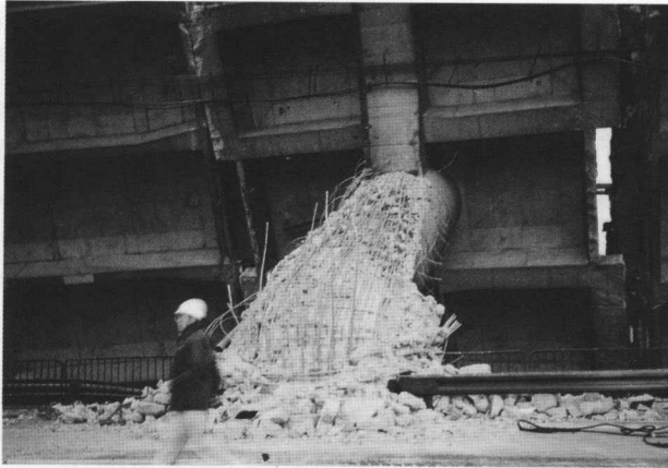
Photo 9 Expressway piers and girders failed and collapsed (PC bridge constructed in 1969, at Fukae honjyo-cho, Higashinada Ward in Kobe city)
